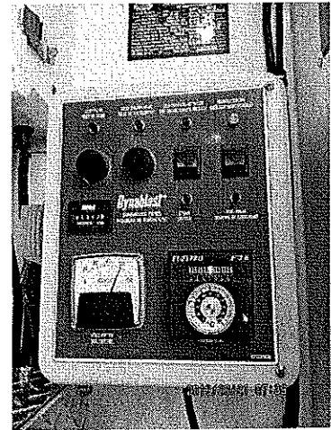
Water Heater control panel located in the van body
